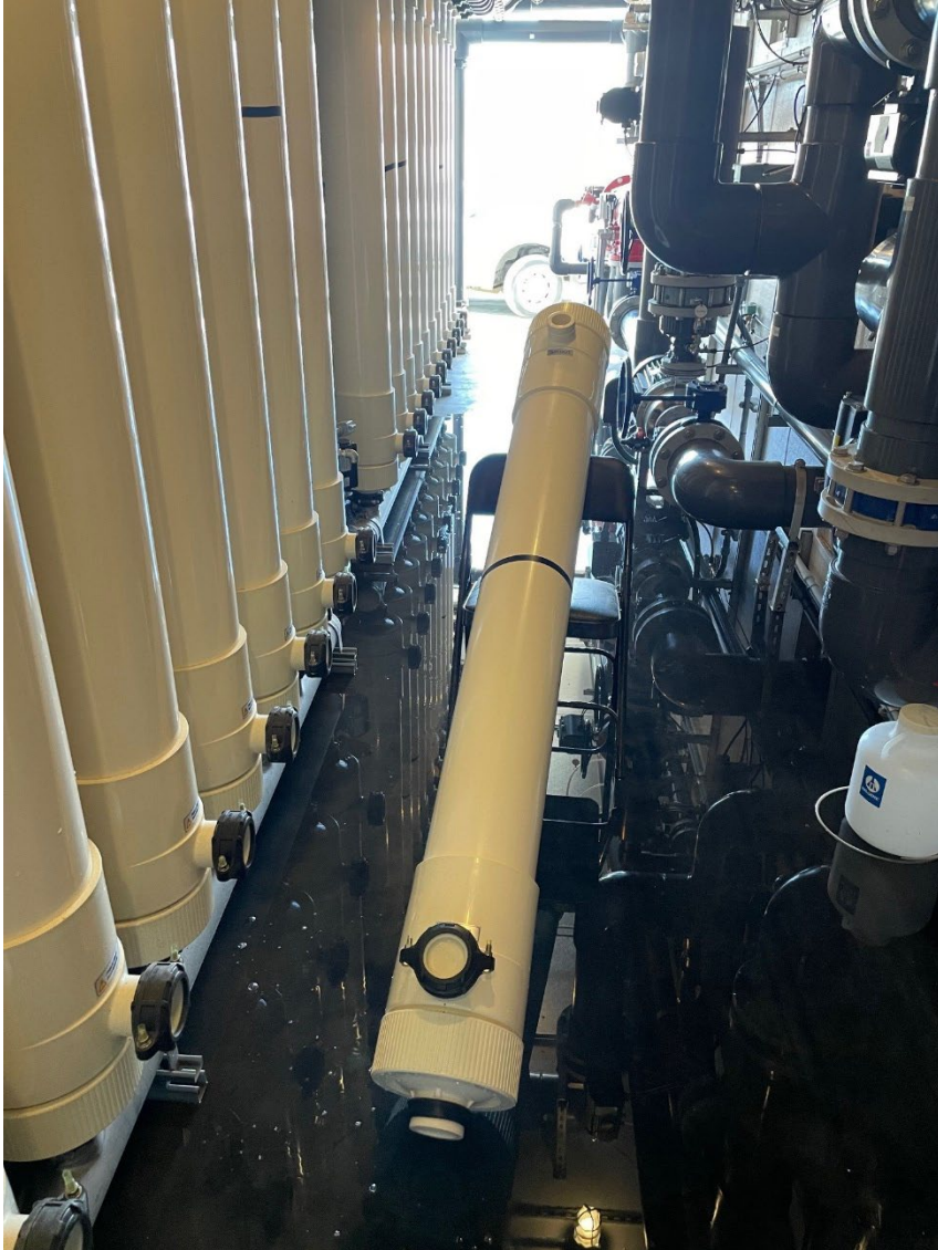
The module was removed, allowing the cap to be removed to gain access to the top Hollow Fibers
