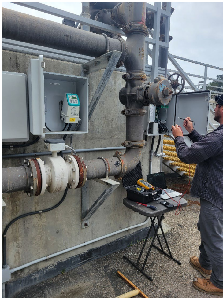
Calibrating WAS flowmeter
