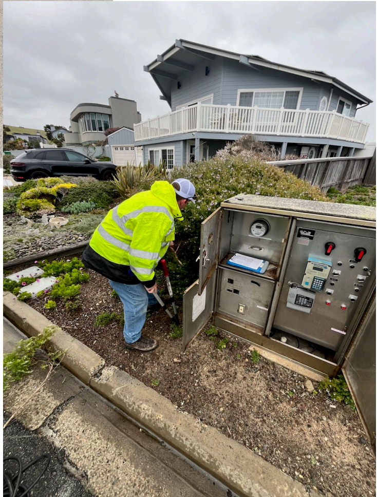
Weekly Lift Station check
