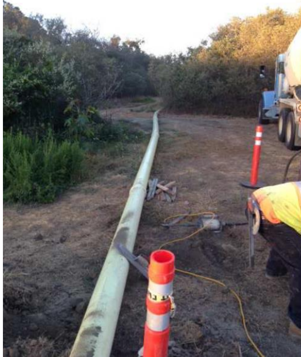
YeloMine Pipe between AWTP and Re-injection Well
