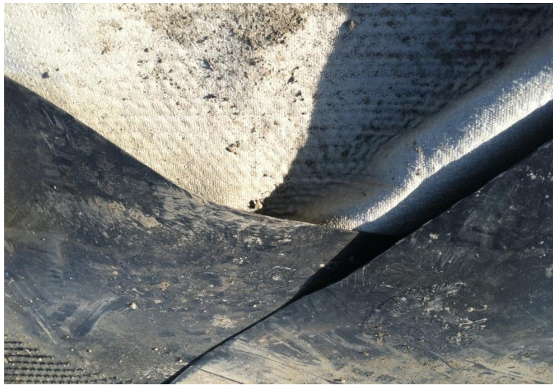
Exposed basin liner close up showing clay liner (white) covered by two 60-mil thick HDPE liners
