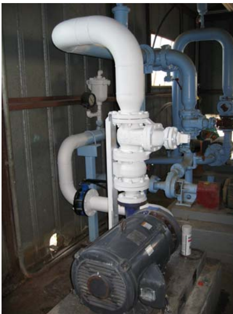
Pump C New Pump and Motor
