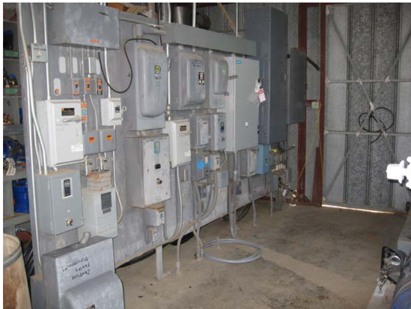
Booster Pump Station Main Power Distribution Panel
