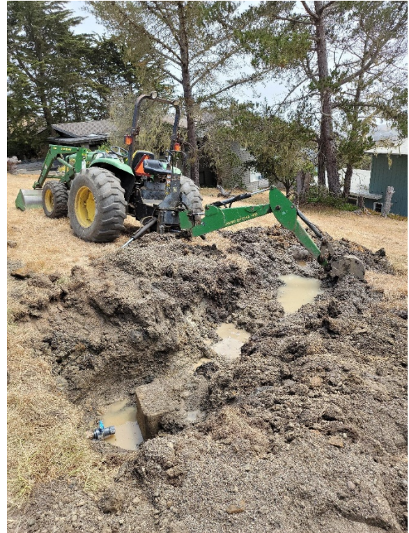
Figure 2 - Blow Off Leak at Victoria Way
