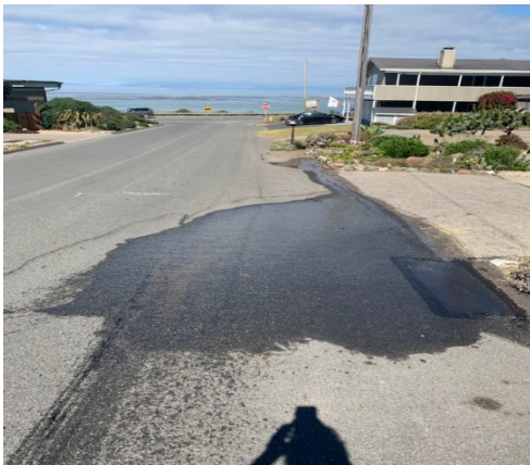
Figure 3 - Distribution system leak on Weymouth
