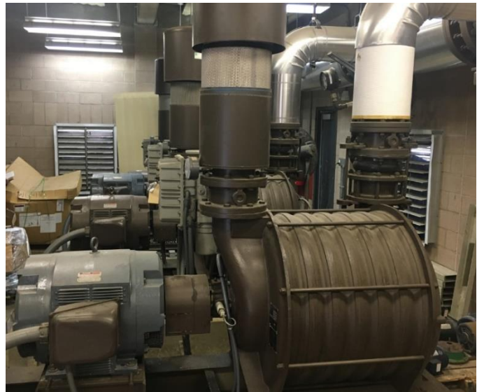
Figure 13: Existing Multi-stage blowers
