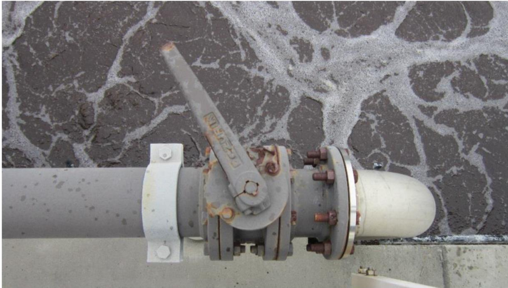
Figure 14: Partially Closed Blower Air Distribution Valve
