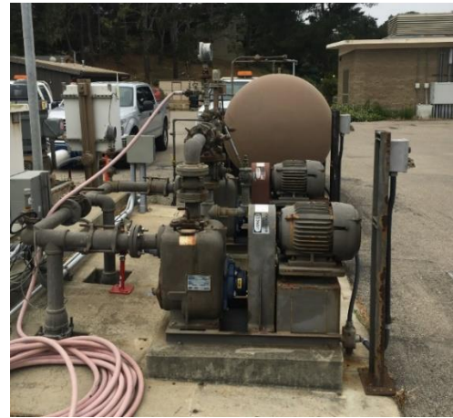
Figure 18: Secondary Water Pump Station
