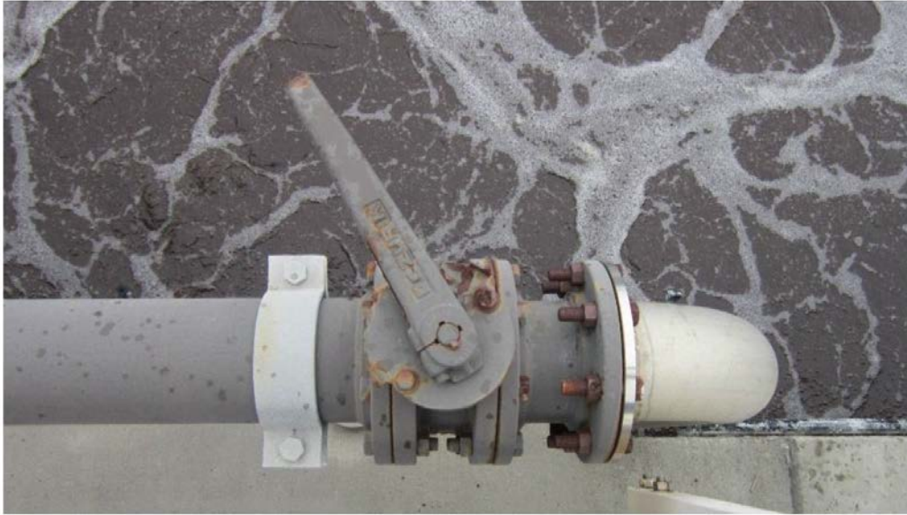
Figure 14: Partially Closed Blower Air Distribution Valve
