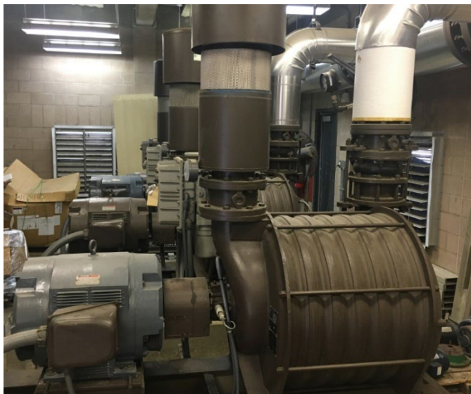
Figure 13: Existing Multi-stage blowers
