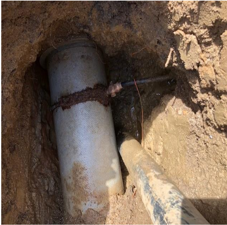
Figure 1 Corroded Saddle on Burton
