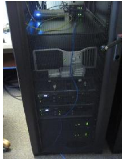
Wastewater SCADA Server
