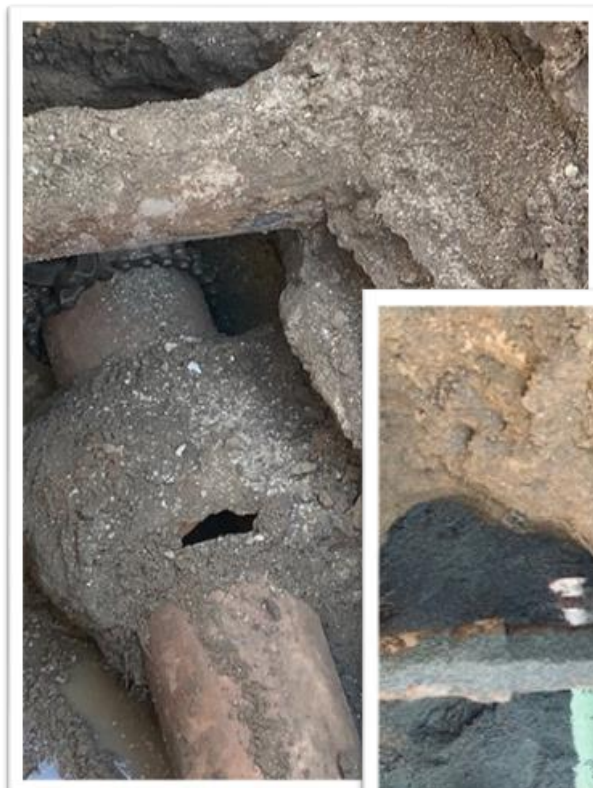
Figure 3 Hole in 8-inch sewer line
