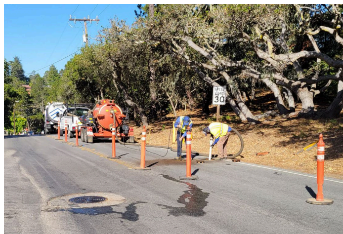
Figure D - Water and Wastewater Crews working together to execute routine maintenance on Ardath Dr
