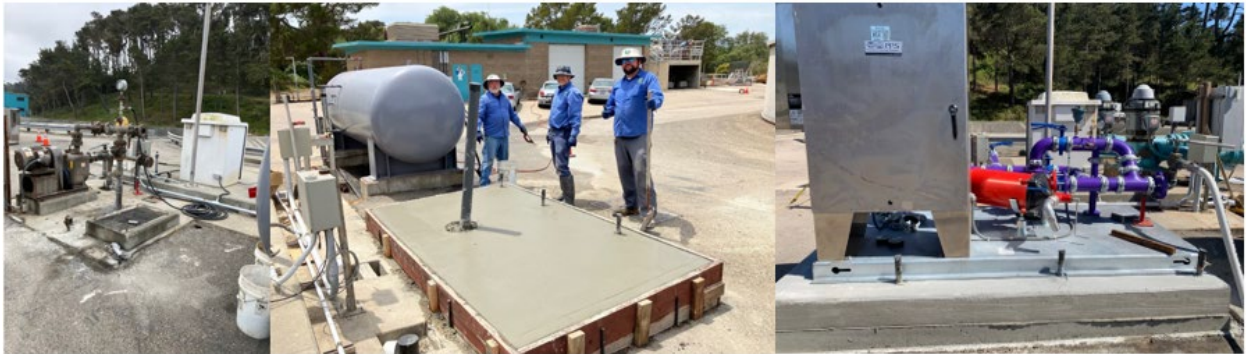
Figure A - Plant water pump pad before (left) and after (middle) staff improvements to prepare for new control center (right)
