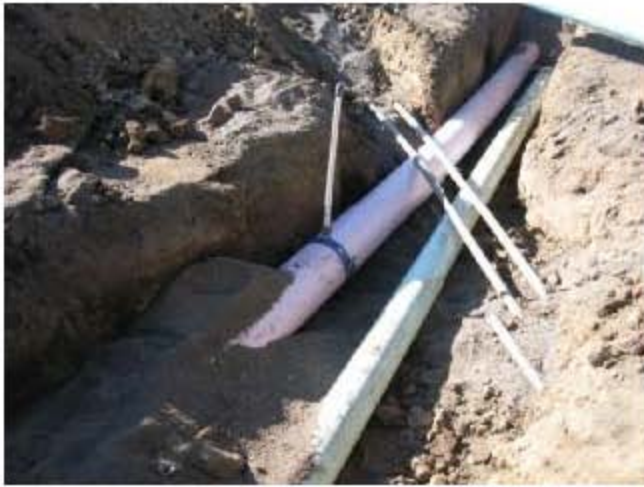
12-inch outfall & 8-inch gravity sewer bypass lines
