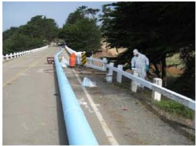
14-inch welded PVC water bypass line
