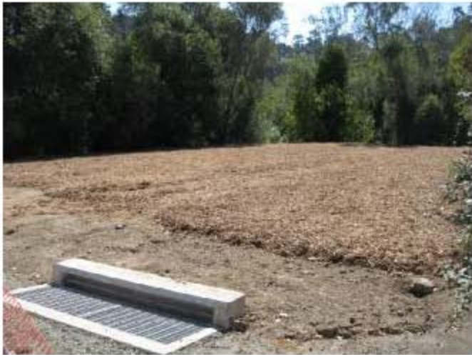
Bridge and Center Street Drop Inlet and Finished Lot After 60-inch HDPE Culver Installation
