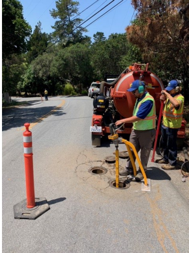
Figure B - Staff exercising valves, and cleaning valve cans in conjunction with hydrant testing.
