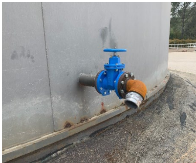
Figure A - Digester valve
