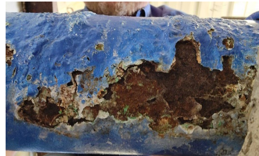
Figure C - Corroded 4" effluent line
