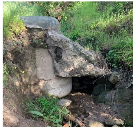
Figure B - Manhole needing repair due to erosion
