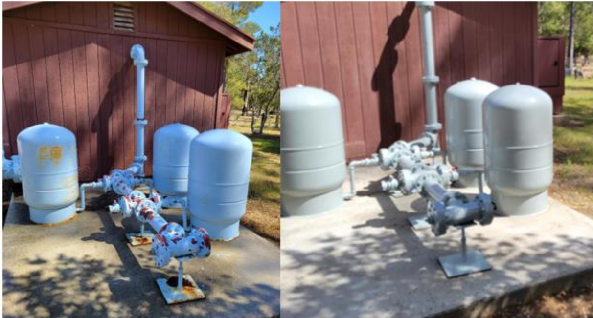
Figure E - Tanks, pipes, and valves before (left) and after (right) painting
