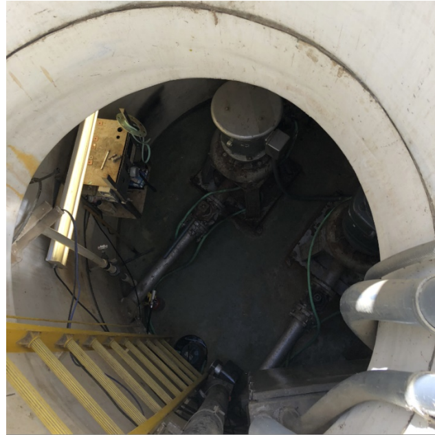
Figure 16: Lift station B4
