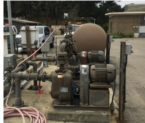
Figure 13: Secondary water pump station
