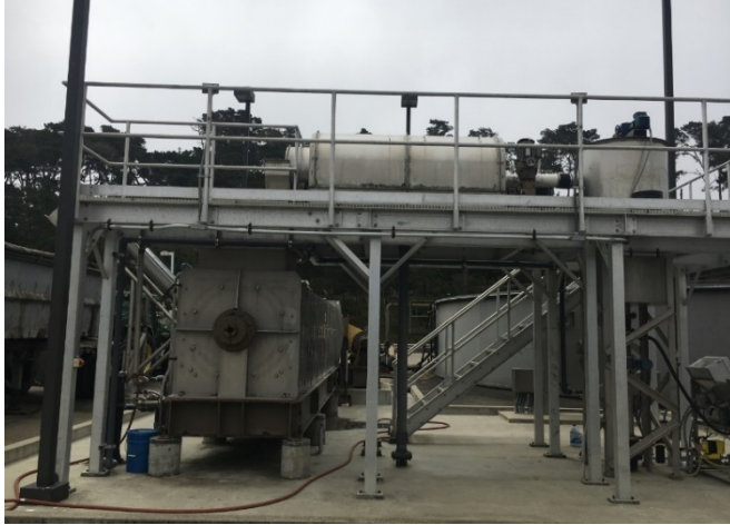
Figure 10: Sludge thickener and screw press
