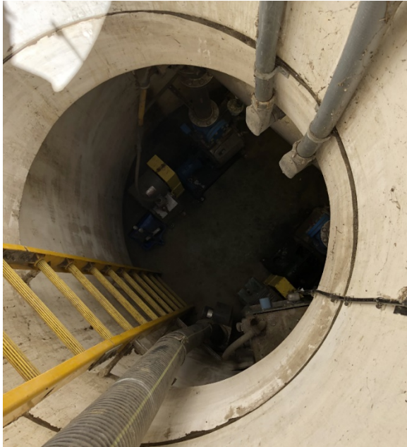
Figure 15: Lift station B1
