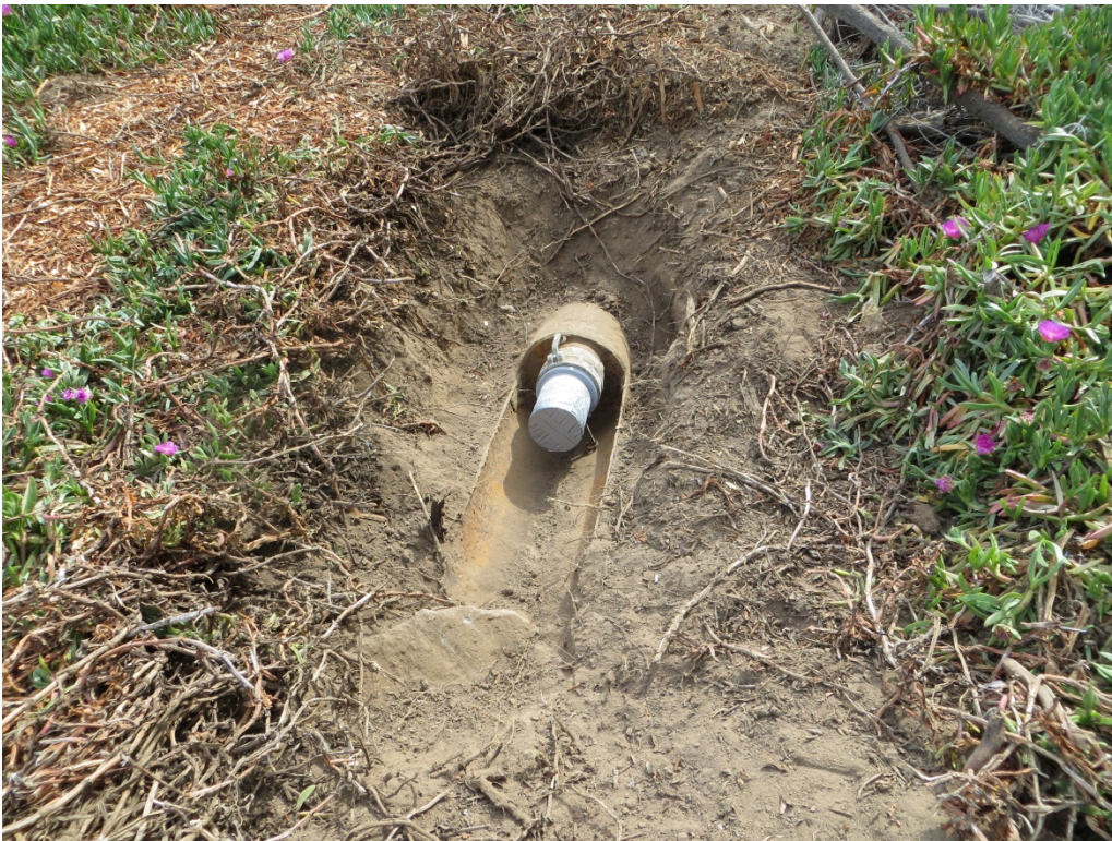
Photograph 8: Facing east. A second alternative for disposing of unusable brine left over from the water treatment is to send it via an existing pipeline to be discharged into the ocean.
