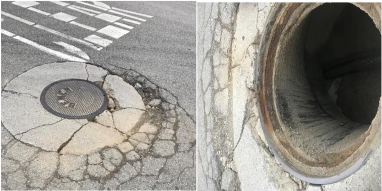
Figure 6 Manhole to be repaired at Main and Windsor
