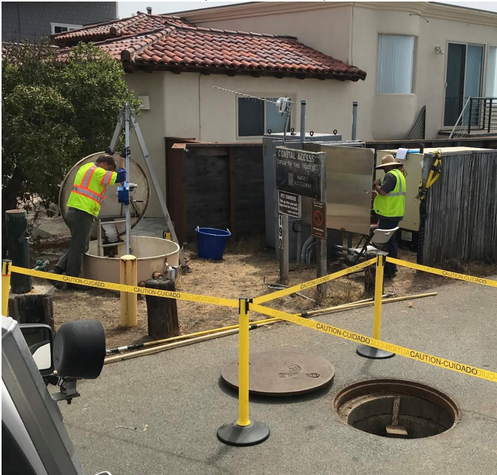
Figure 7 New control panel
