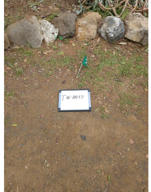
Manhole TW-10057 was covered up and needs to be raised to the ground level.
