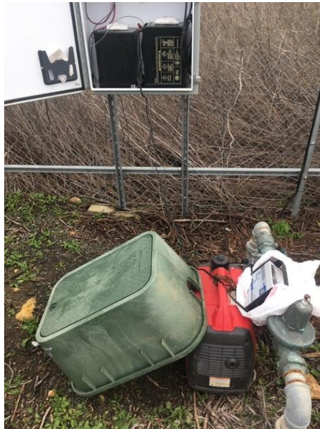
Figure 3 Temporary power setup for communications at SS/SWF SCADA Relay Station
