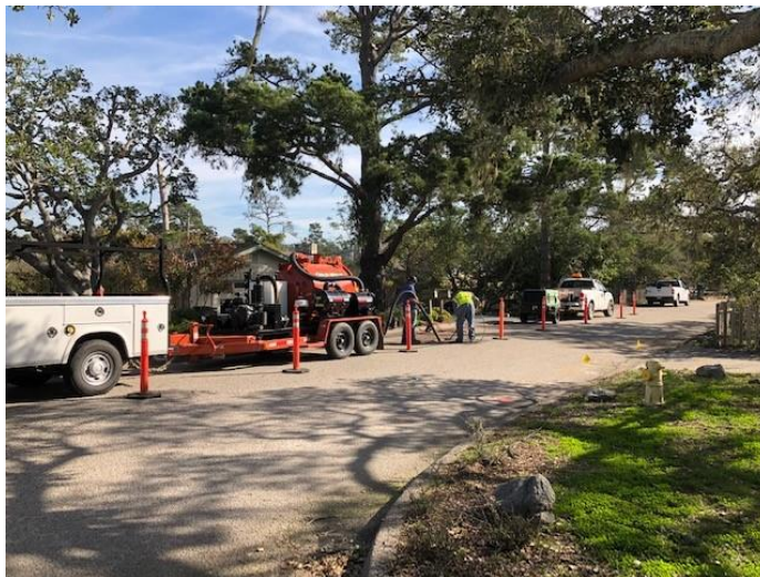
Figure 2 Service line repair on Hillcrest using vacuum excavation trailer—a very helpful tool for reducing time on site and protecting staff from injury.
