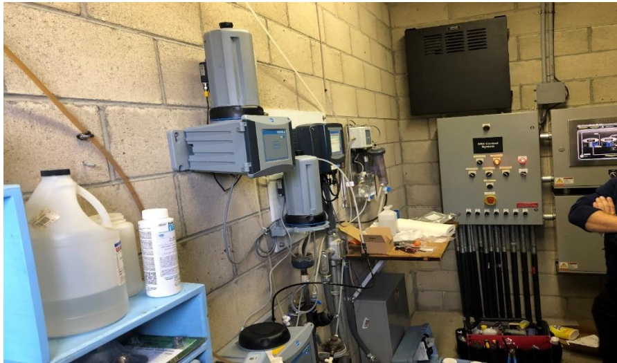
Figure 1 New turbidimeter installation at SR4
