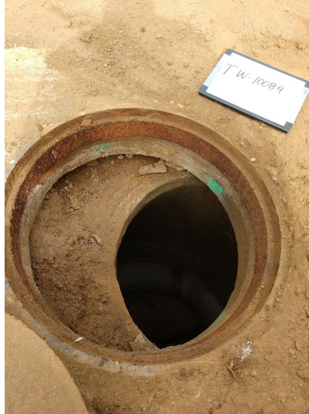
Manhole cover TW-10084 was damaged and needs to be replaced.
