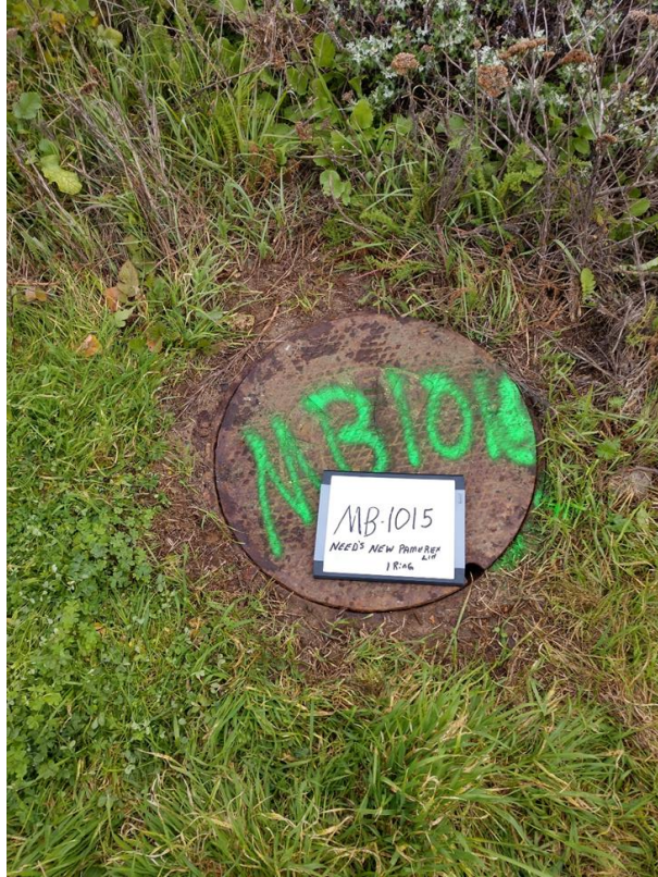
Manhole MB-1015 floods when it rains and needs to be replaced.
