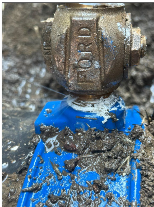
4. Saddle and shutoff with the leak visible in the middle of the picture
