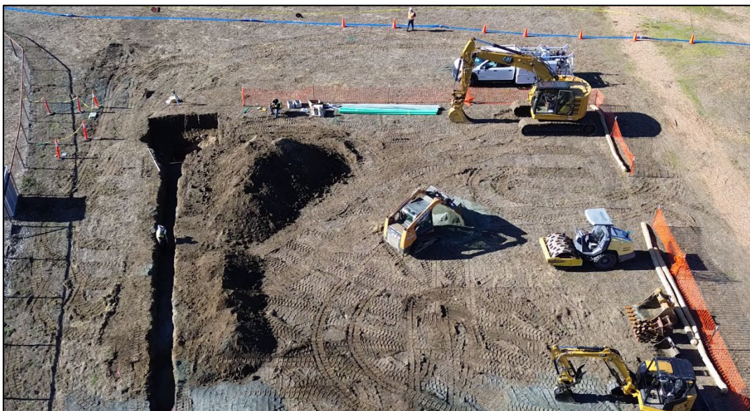
1. East Ranch Restroom construction site. The sewer lateral trench is on the left and the bypass hose is just visible as the blue line across the top of the image
