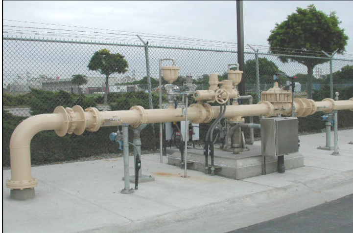
Figure 3.2.5-7 Wellhead of Typical Injection Well
