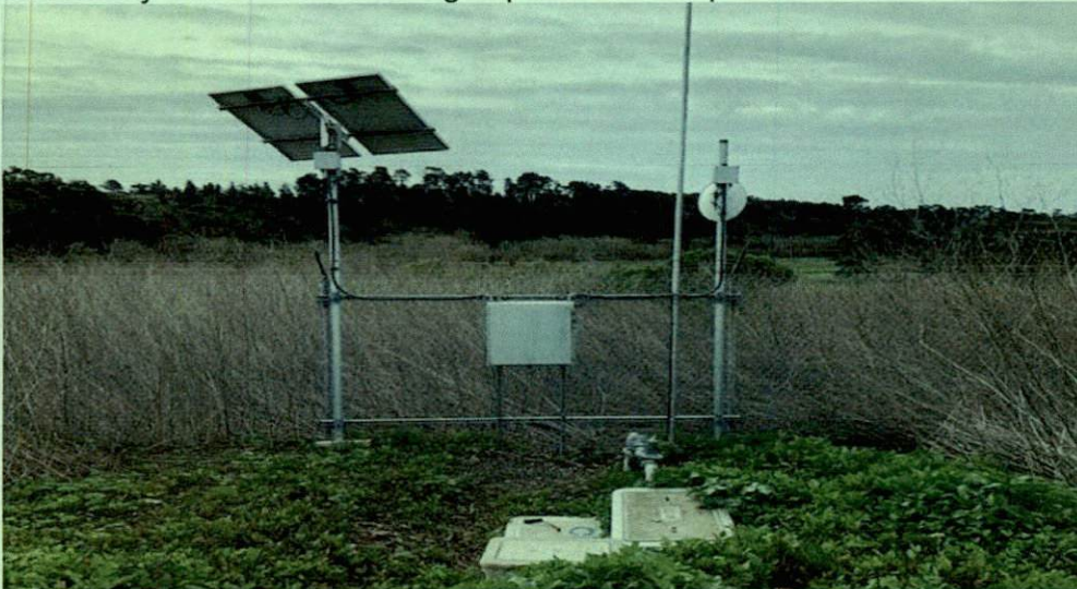
Relay Station at San Simeon Well Field
