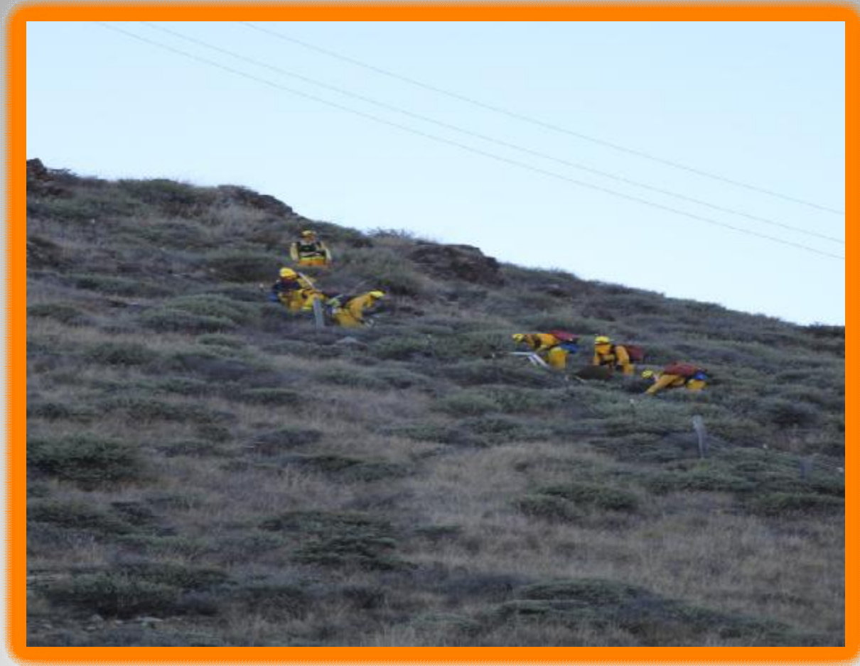
1100 foot - Progressive Hose Lay
