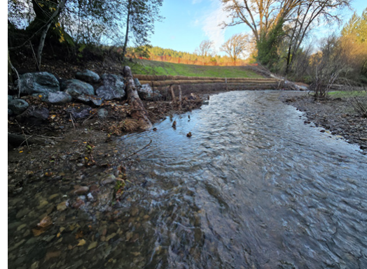
Streambank restoration on Tenmile Creek. This photo highlights Stillwater’s engineered design in action. The bioengineered coir soil lifts and strategically placed boulder/large wood structures replace traditional rock armoring to stabilize eroding banks and create critical habitat for ESA-listed salmon and steelhead. See References for more information on this project.
