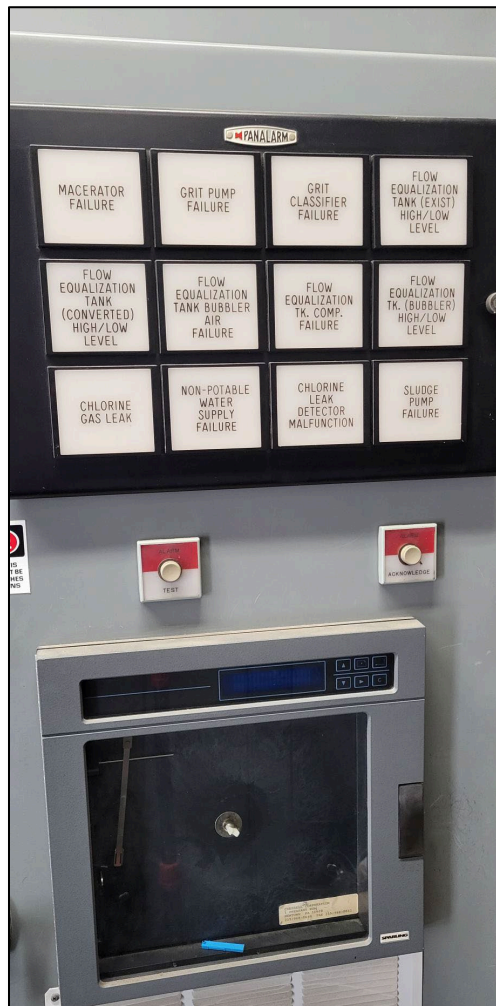
Figure 8: 1980's Era Analog Control Panel
