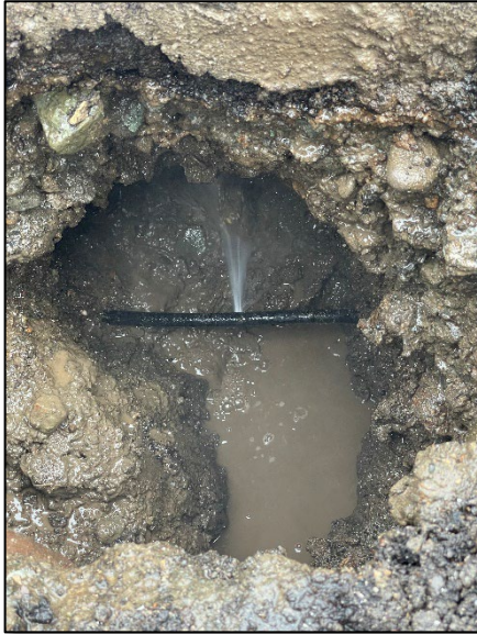
Figure 16: Main Street Water Leak
