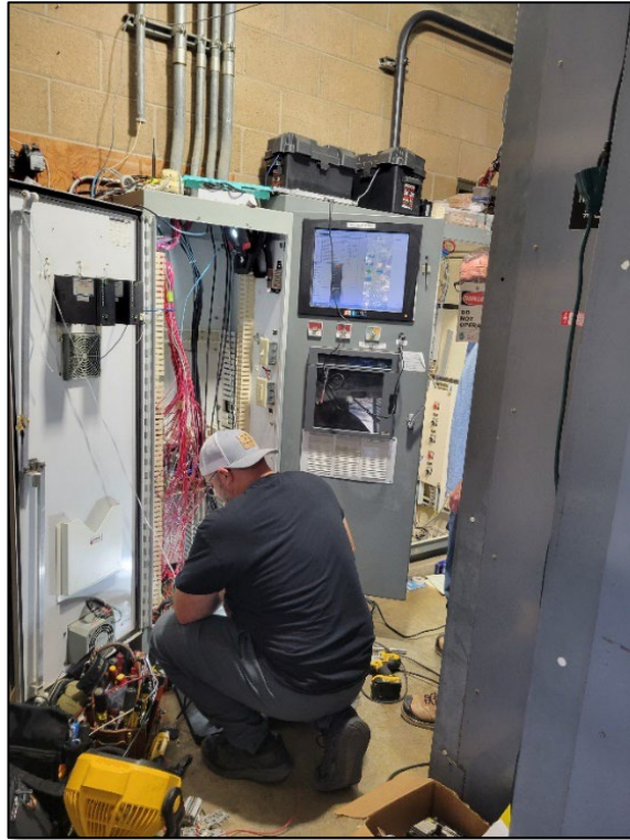
Figure 5: Tough Automation Updating System Wiring
