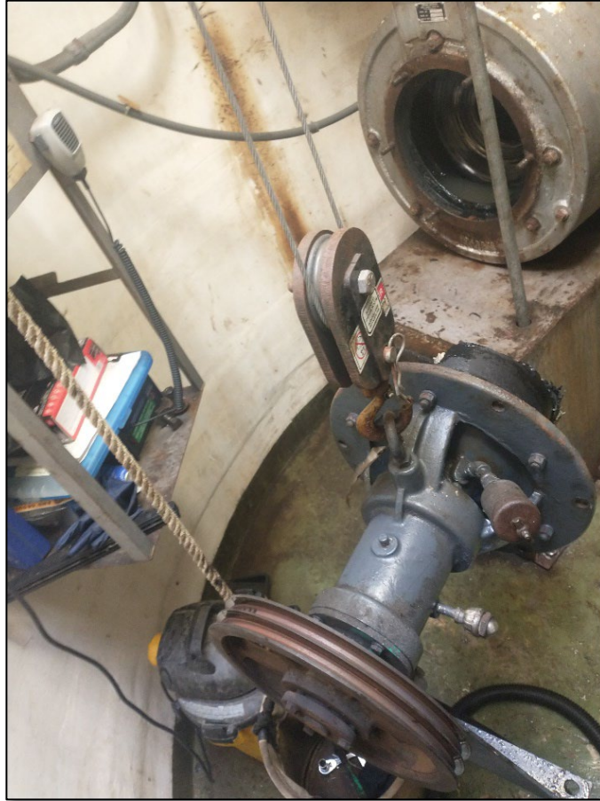
Figure 11: Rotary Assembly From Lift Station A
